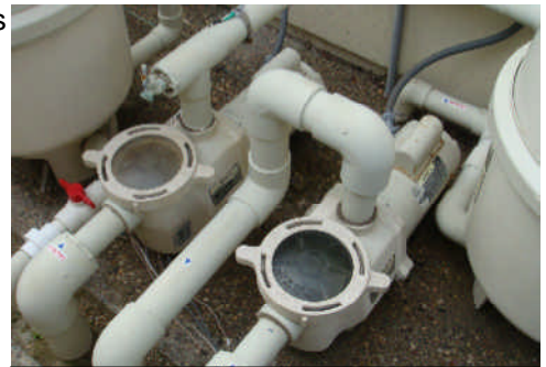
Spa booster pump and filter pump.
