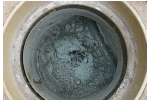
Skimmer basket missing.
