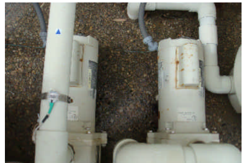
One or two pumps suspected leaks.
