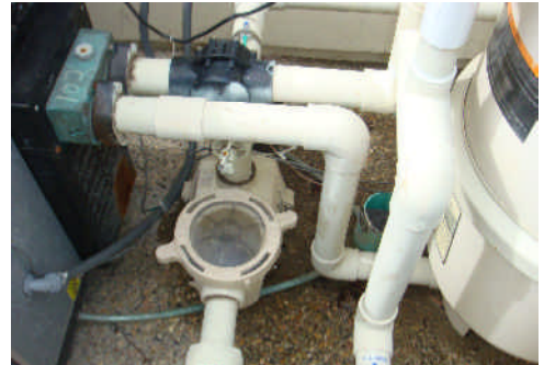
Pool filter pump.
