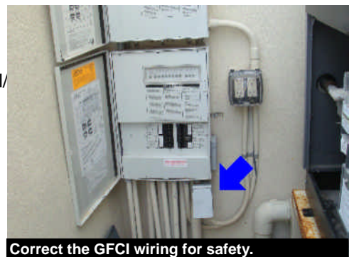
Correct the GFCI wiring for safety.
