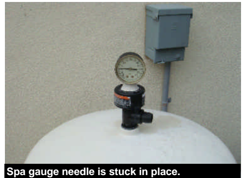
Spa gauge needle is stuck in place.
