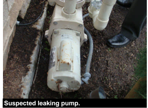
Suspected leaking pump.
